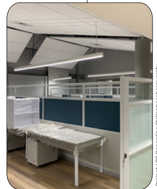
Project LGS Decating Stellenbosch University
